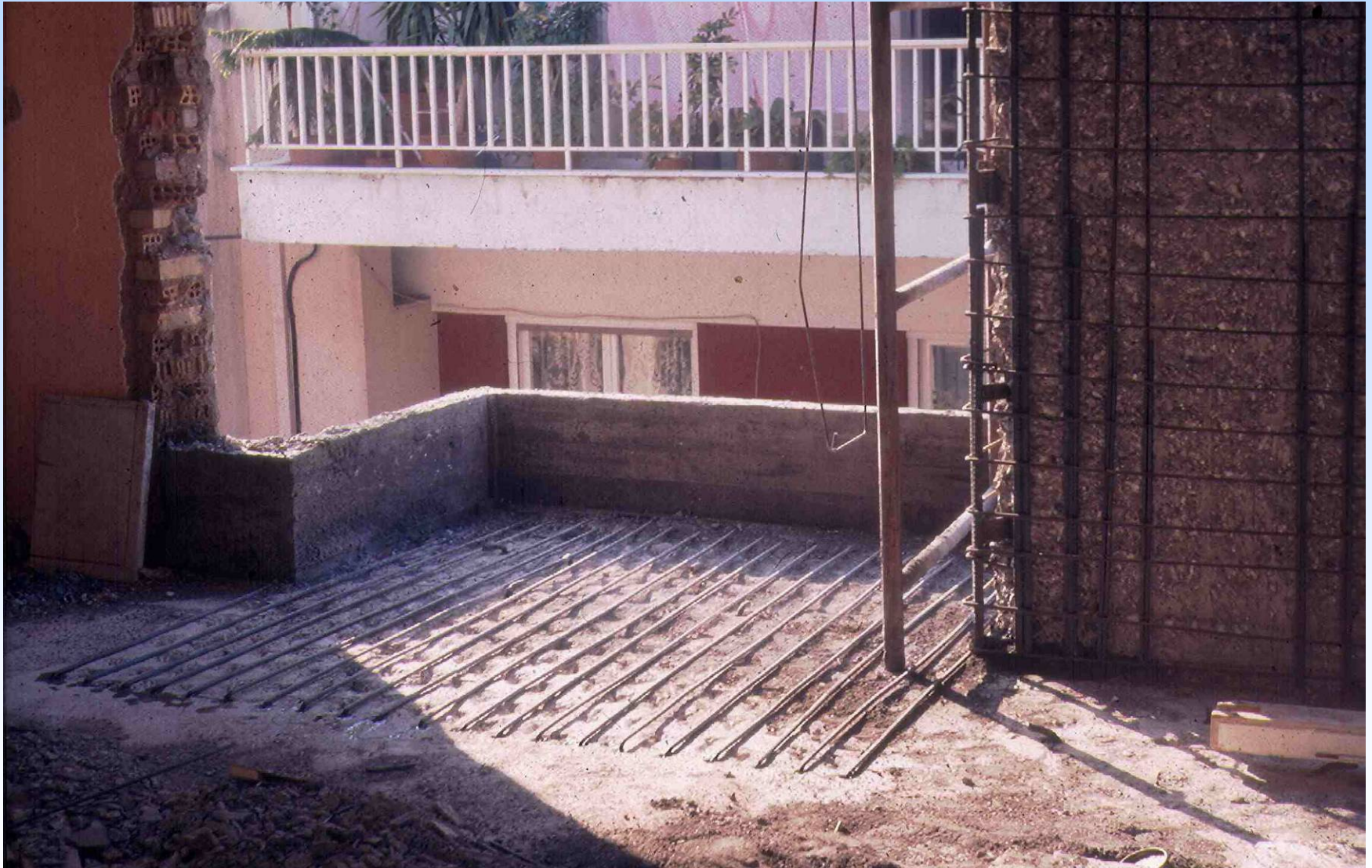
Addition of a new concrete layer to the top of a cantilever slab
