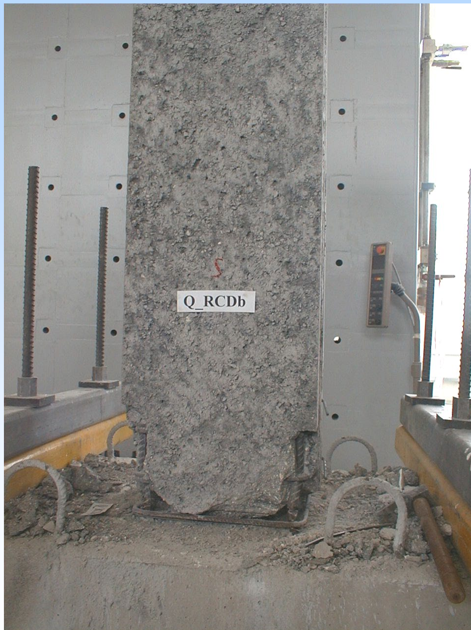
Damage to a specimen with shotcrete and dowels
