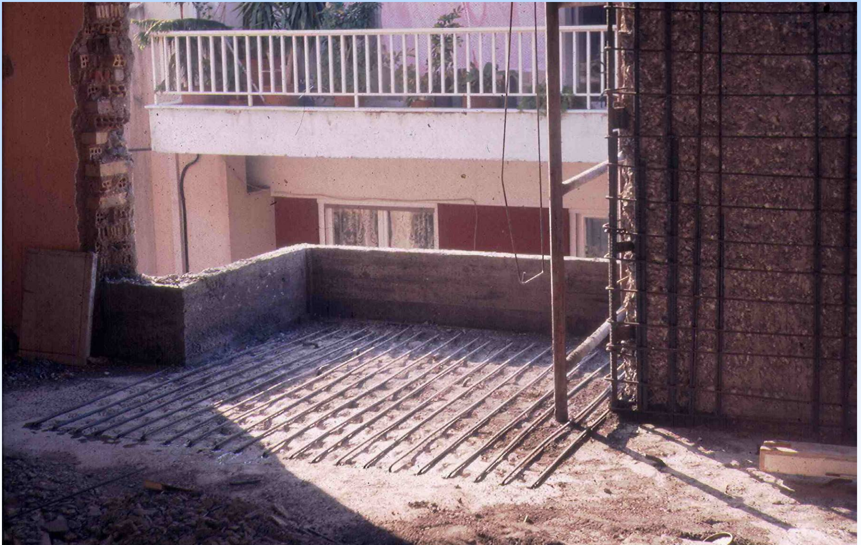
Addition of a new concrete layer to the top of a cantilever slab
