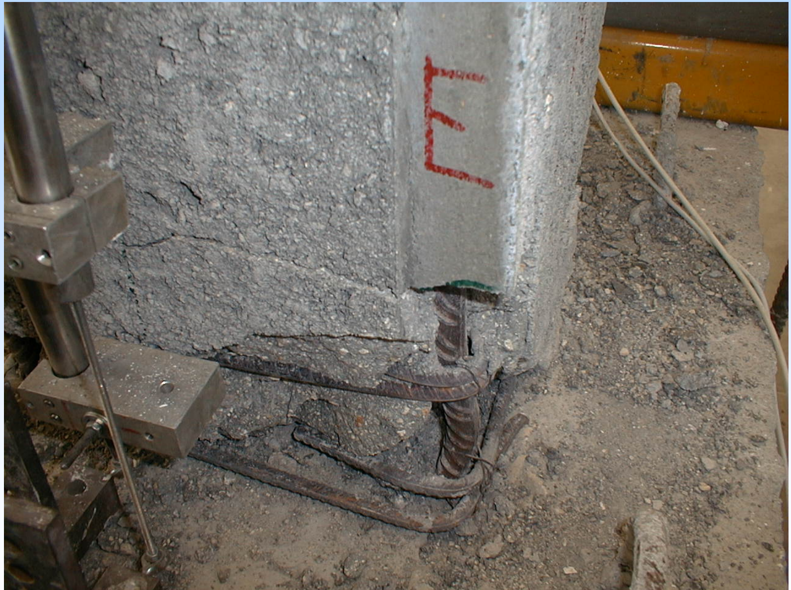
Bar buckling due to stirrup ends opening
